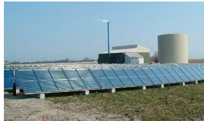
Nordby 2 500 m 2 / 1,8 MW Combined with wood chip boiler
